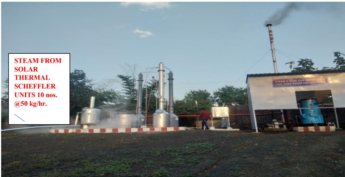
Figure 1: A View of Pilot Plant Integrated with Solar Thermal Steam Generator & A Coal Fired Boiler for Production of CO 2
