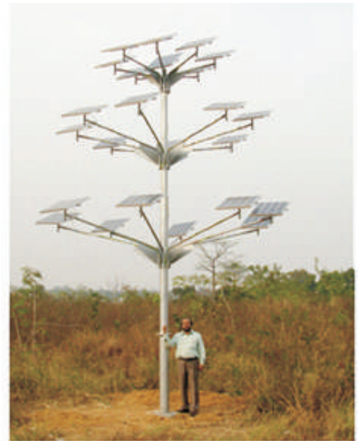
A Solar Power Tree
