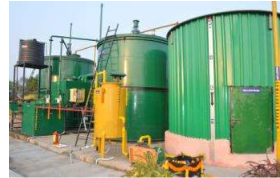
Bio-gas plant at Paradip Refinery Township
