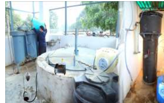
50 kg/d Bio Gas plant at IOC R&D
