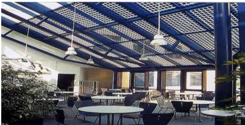
Roof Integrated Solar Photovoltaic
